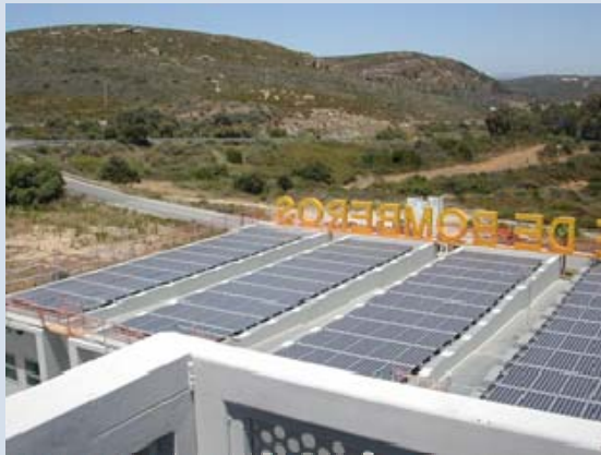
SAN ROQUE 50 kW
