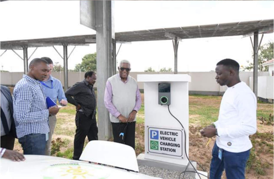
EV-chargers /Powered by solar system UNDP-Dodom
